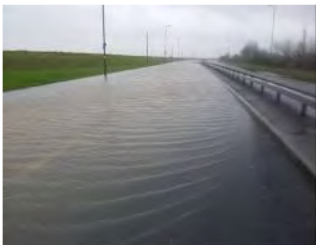
Photo 1: Tidal flooding A2030 January 2014
